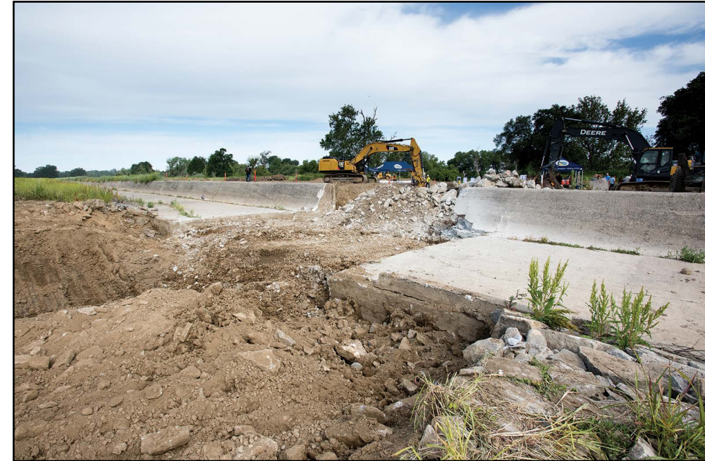
In this photo taken May 30, 2018, an excavator has broken up a section of the Fremont Weir for the Adult Fish Passage Modification Project, to restore an important migration corridor for native fish species and fulfill requirements set forth in the 2009 National Marine Fisheries Service's Biological Opinion. California Department of Water Resources (DWR), U.S. Bureau of Reclamation, California Natural Resources Agency and other federal, state, and local partners celebrate the groundbreaking of the Fremont Weir Adult Fish Passage Modification Project, a critical habitat improvement project in the Yolo Bypass. Source: Department of Water Resources
