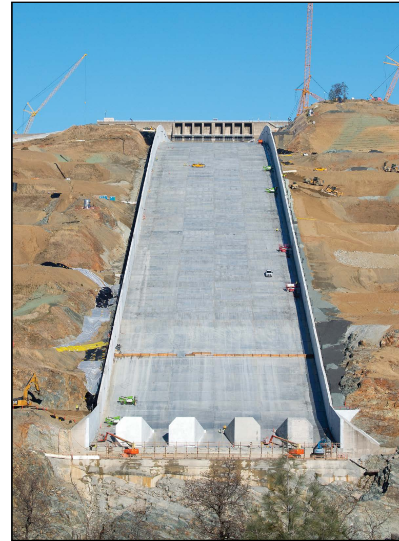
In this photo taken December 10, 2018, cleanup work continues along the Lake Oroville main spillway in Butte County. Source: Department of Water Resources
