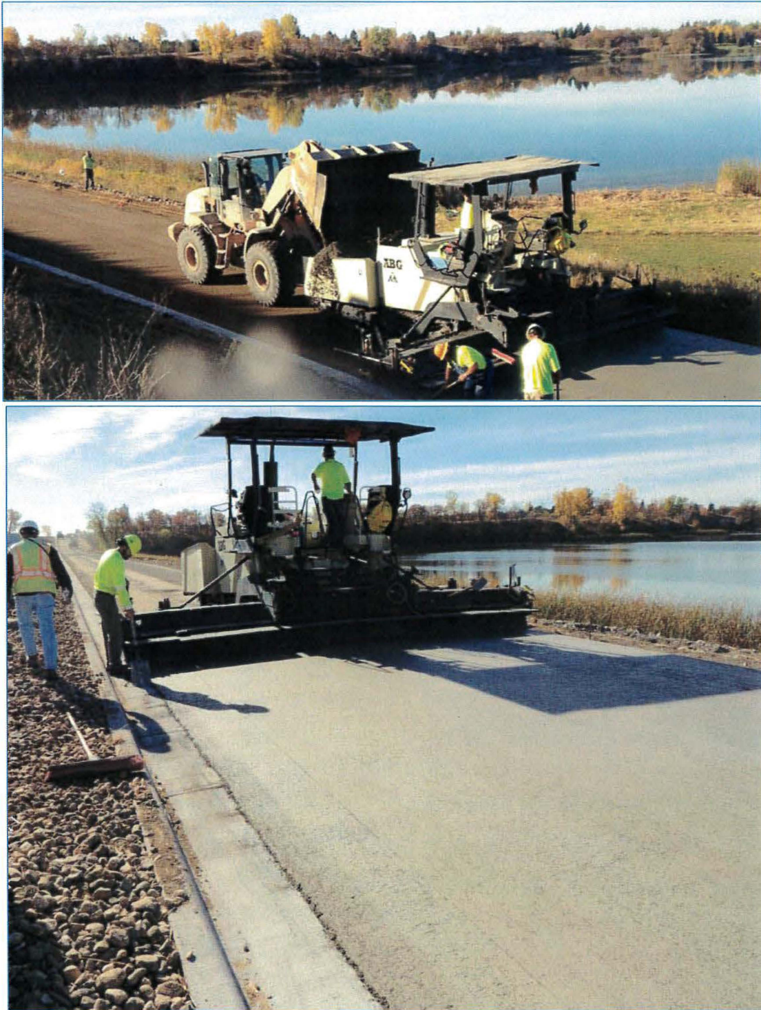
Figure 1. Photographs showing placement of RCC using a conventional mechanical paver machine at Renwick Dam at Icelandic State Park in North Dakota.
