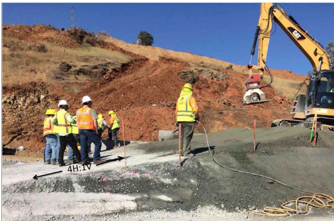
Figure 4. Photo of the 4H:1V ramp on the RCC Test Section that is planned to be formed by vibratory rollers.
