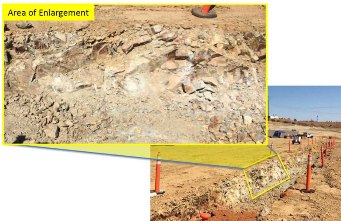
Figure 2. Photo of moderately weathered amphibolite rock exposed in a portion of the secant guide wall trench near approximate Station 17+00.
