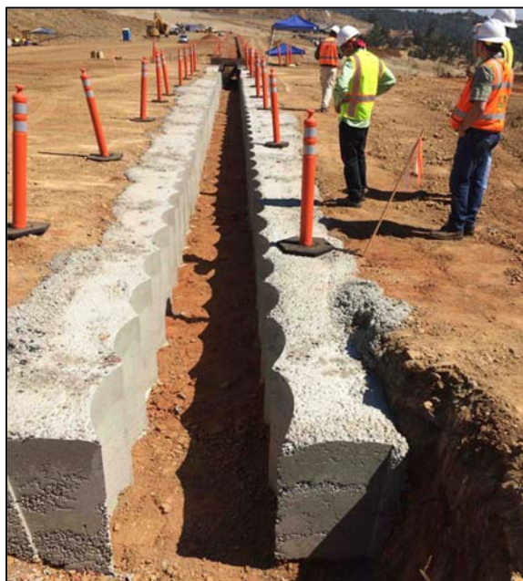
Figure 1. Photo of secant guide wall trench at approximate Station 13+00. View to the south.
