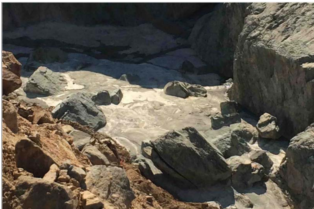
Figure 5. Flowable fill that has been placed in the scour hole near approximate Station 32+00.
