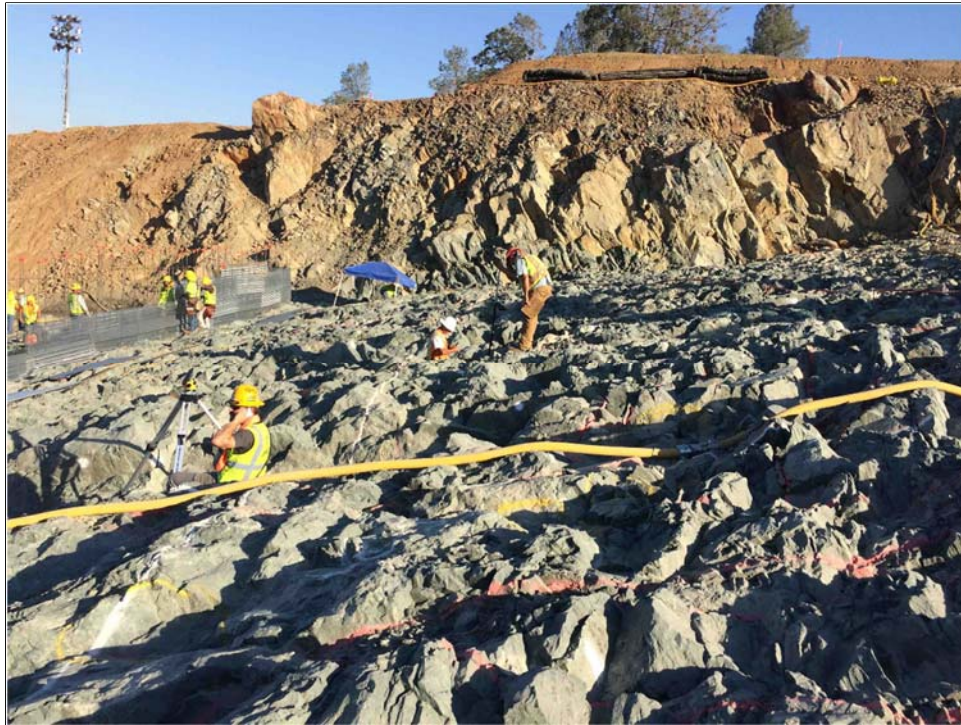
Figure 6. Cleaned FCO spillway chute rock that has been geologically mapped and is close to being accepted for concrete placement. Near approximate Station 33+00.
