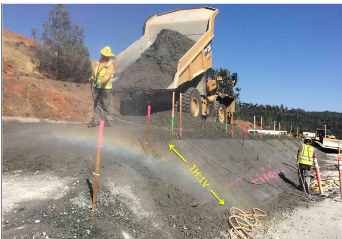
Figure 3. Photo of RCC placement of lift 8 and the vibratory finish of the 1H:1V slope.
