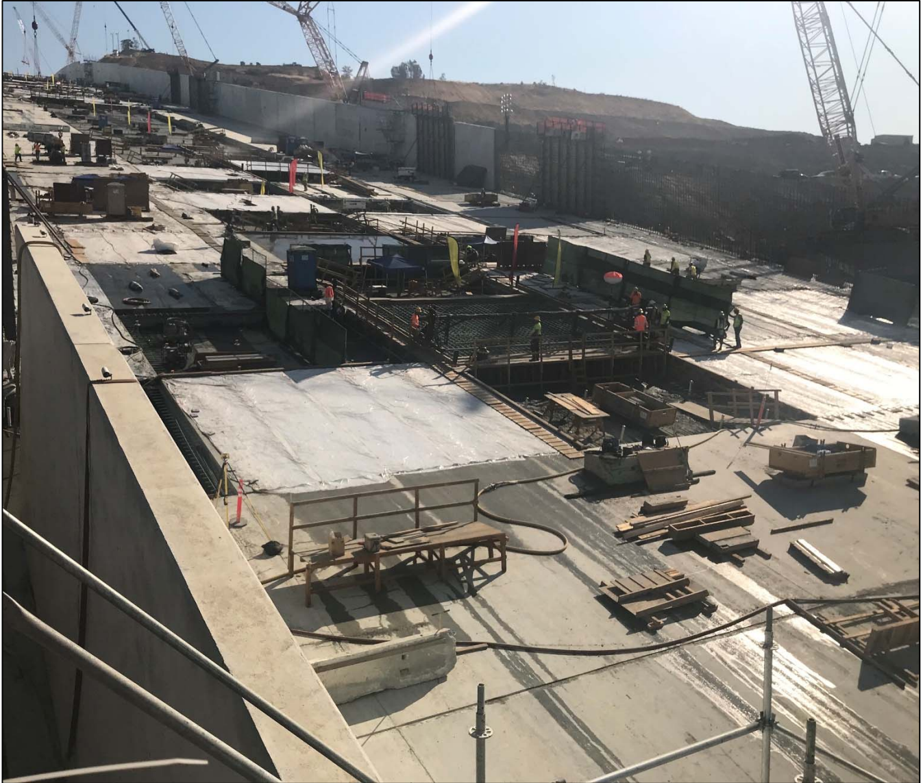
Figure 2. Construction of chute slabs and walls in the middle section of FCO chute.
