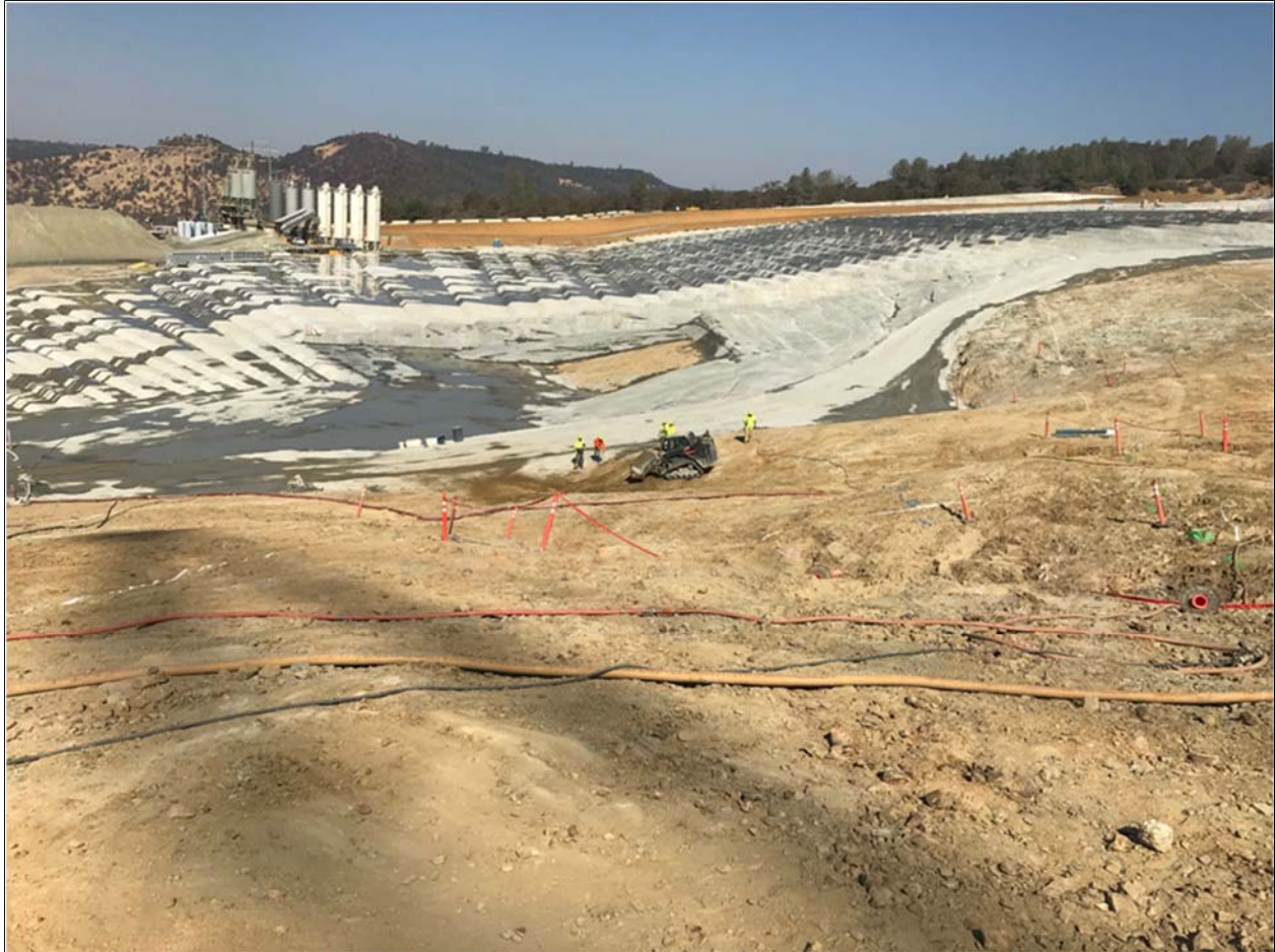
Figure 6. View of Emergency Spillway completed Areas 1 and 2A. Area 2B is the foreground area.
