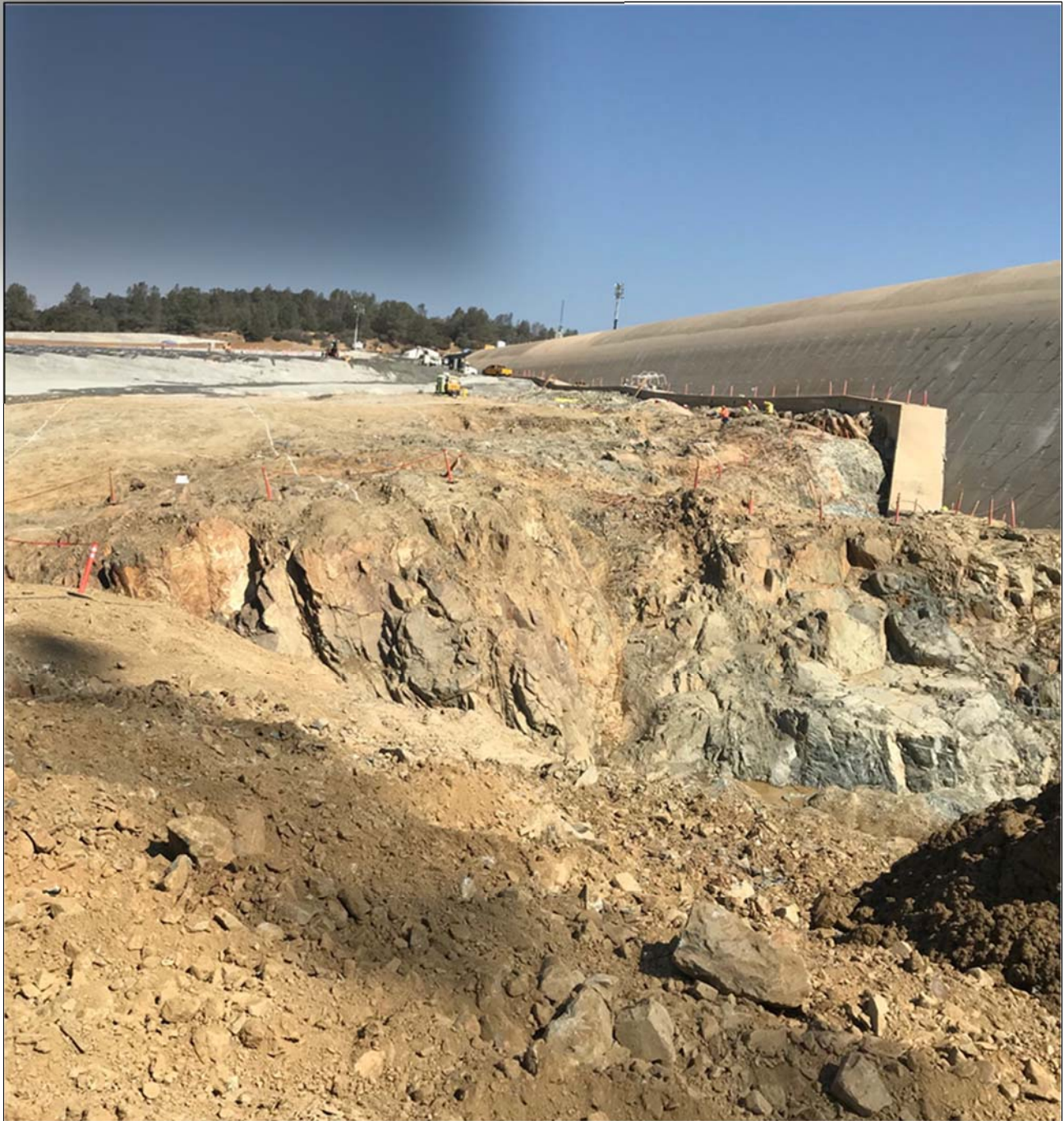
Figure 5. Final excavation and foundation preparation for the RCC apron and RCC buttress on the left side of the Emergency Spillway
