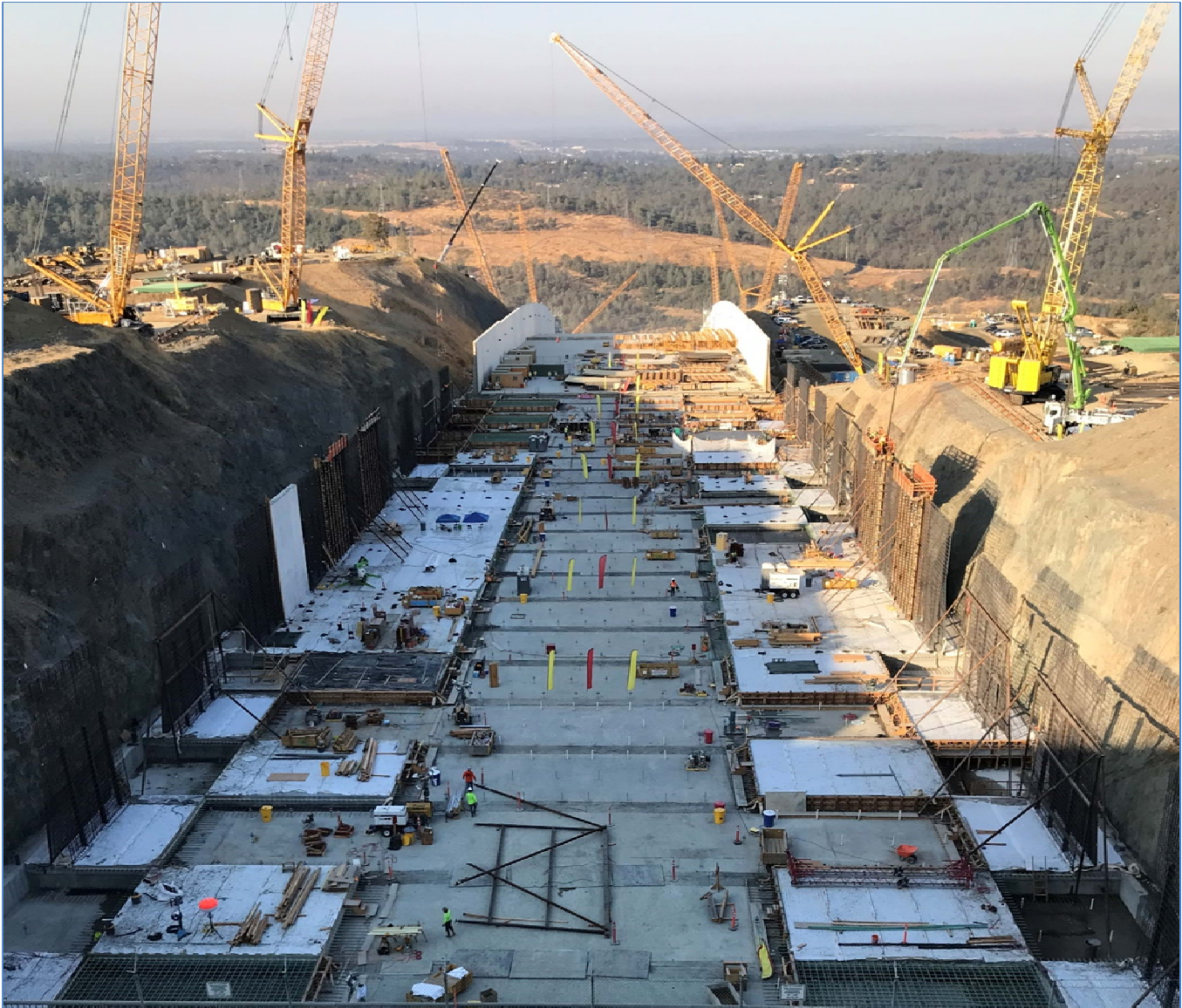
Figure 1. Construction of chute slabs and walls in the upper section of FCO chute.
