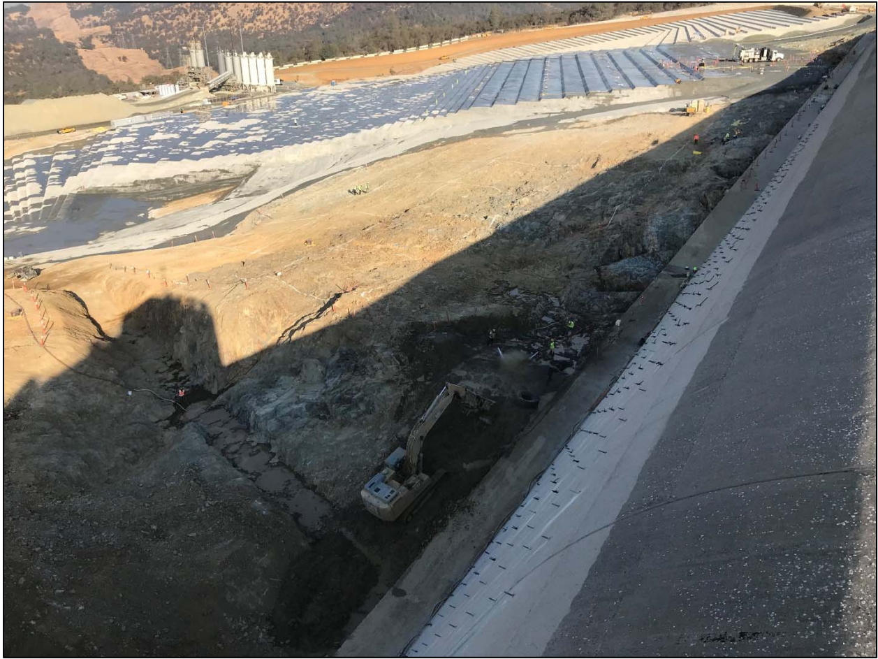
Figure 4. Final excavation and foundation preparation for the RCC apron on the left side of the Emergency Spillway.
