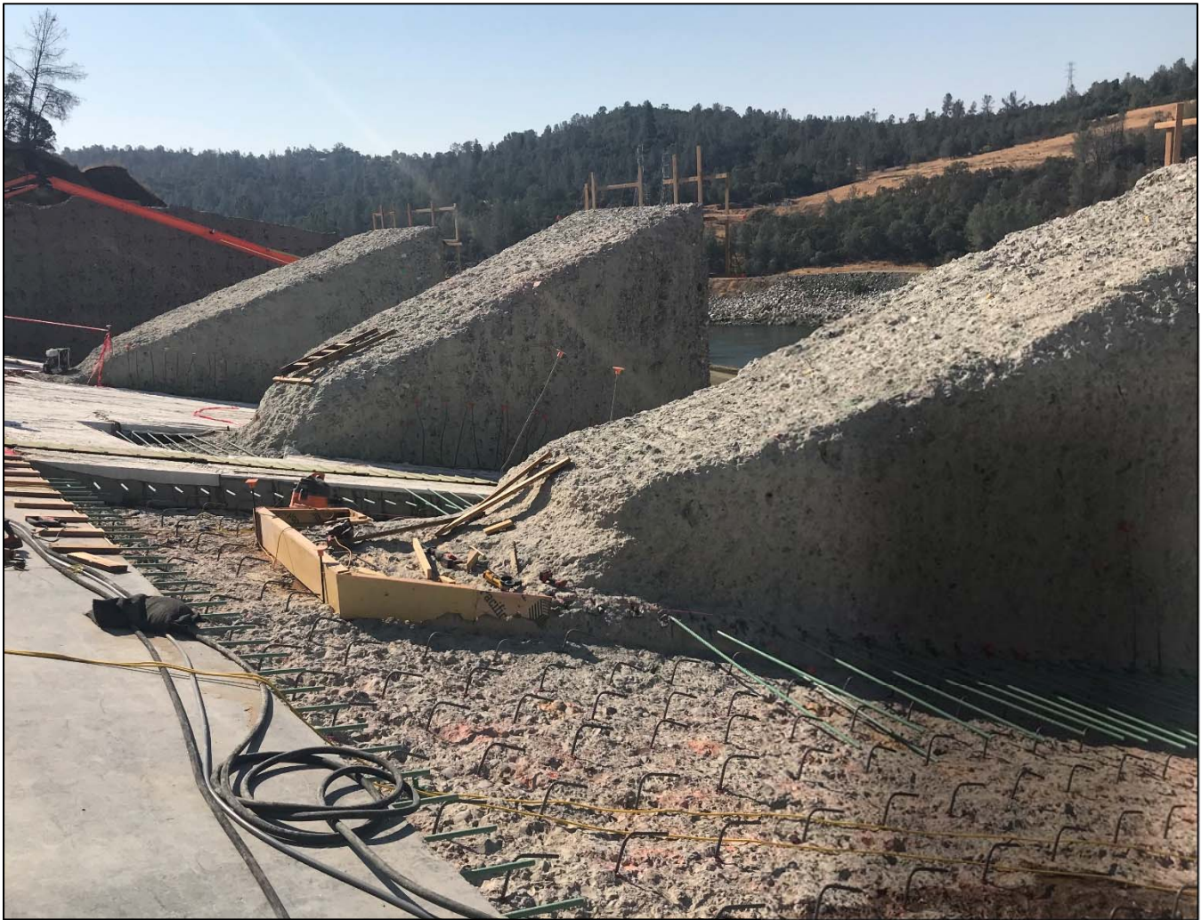
Figure 3. Final surface preparation and initial placement of reinforced concrete to rehabilitate the FCO terminal structure. Photo inset shows concrete spall on the downstream face of a dentate.
