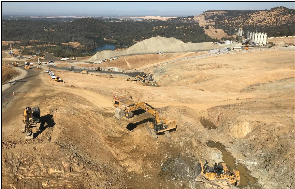
Figure 3. Photos showing FCO dentates and left side of Emergency Spillway RCC foundation preparation.
