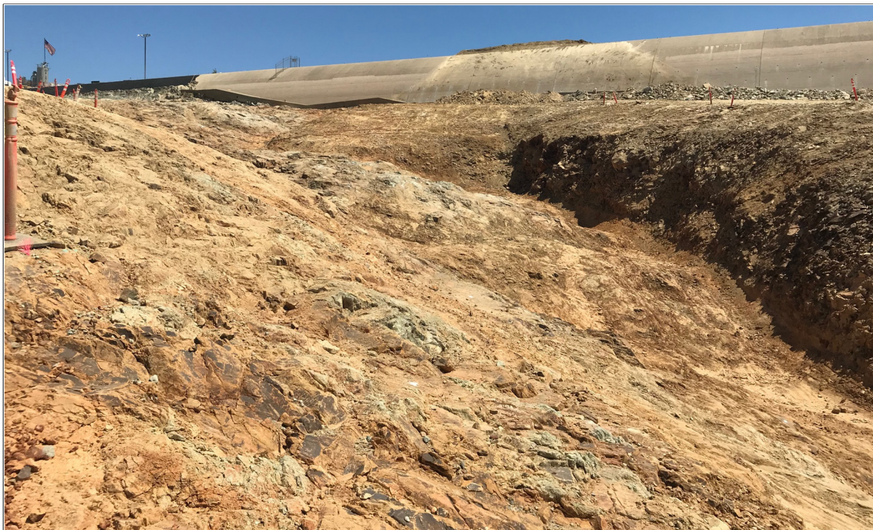
Figure 5. Erosional channel in Emergency Spillway apron foundation that will be filled with backfill and RCC concrete
