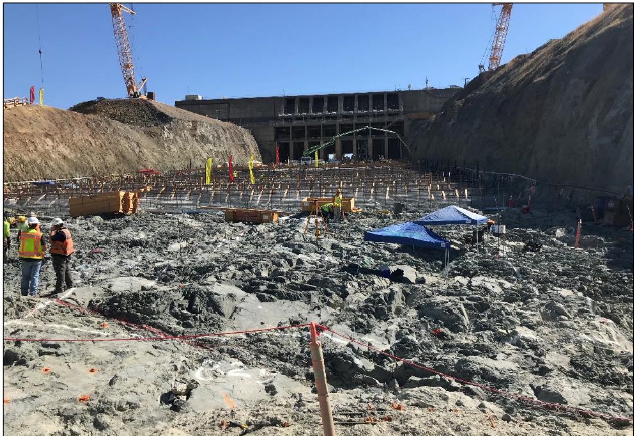
Figure 1. Photos of the foundation preparation at the upper section of the FCO chute.
