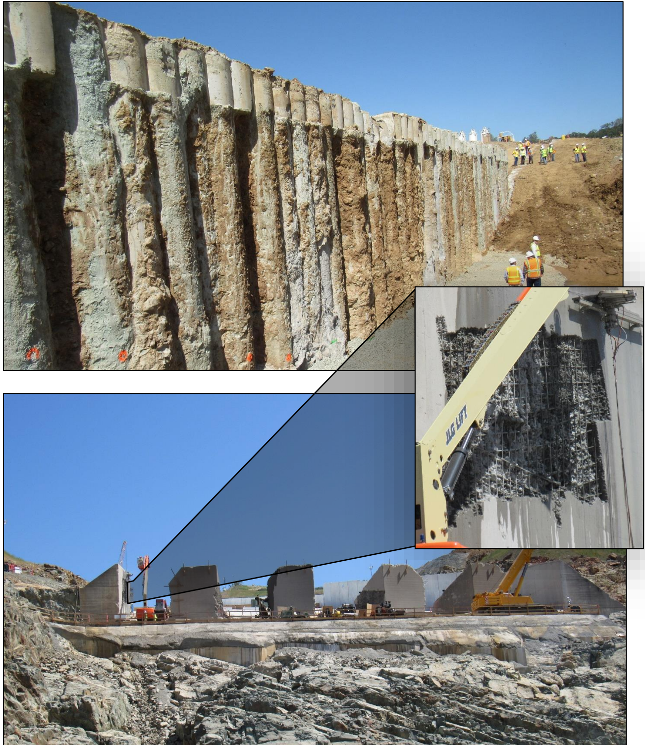
Figure 2. Photographs showing exposed secant pile cutoff wall at left side of the Emergency Spillway (Top) and Hydro-demolition work for rehabilitation of the Dentates at the downstream end of the FCO Chute
