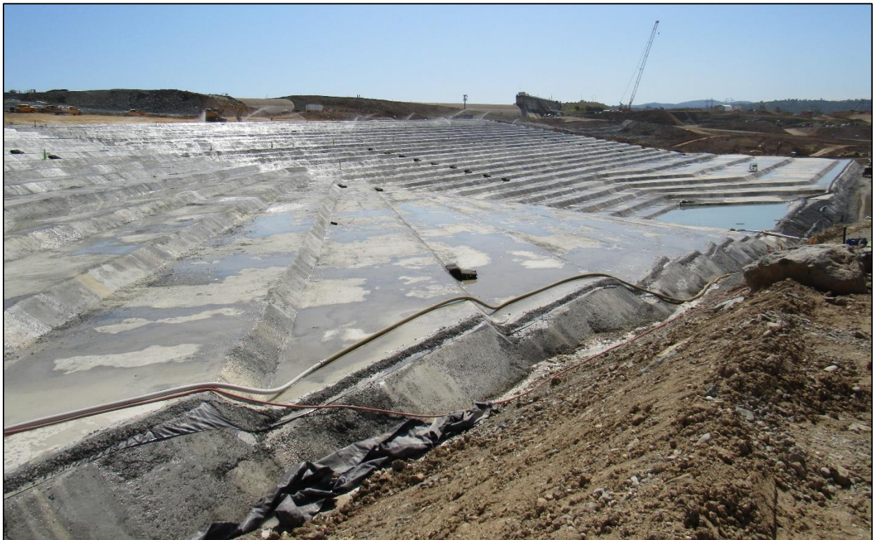
Figure 1. Aerial photographs of the Emergency Spillway Construction (Top), and Emergency Spillway RCC Apron Construction (Bottom)
