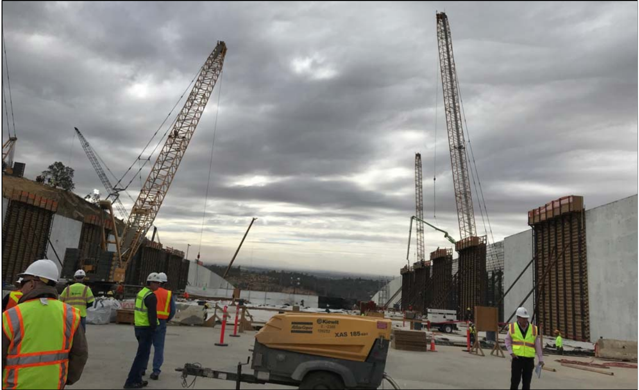
Figure 2. Photograph from the upper FCO Spillway looking downstream. Replacement of the permanent FCO structural concrete walls and chute slab is about complete with all of the floor slabs and all but 8 of the wall sections installed.
