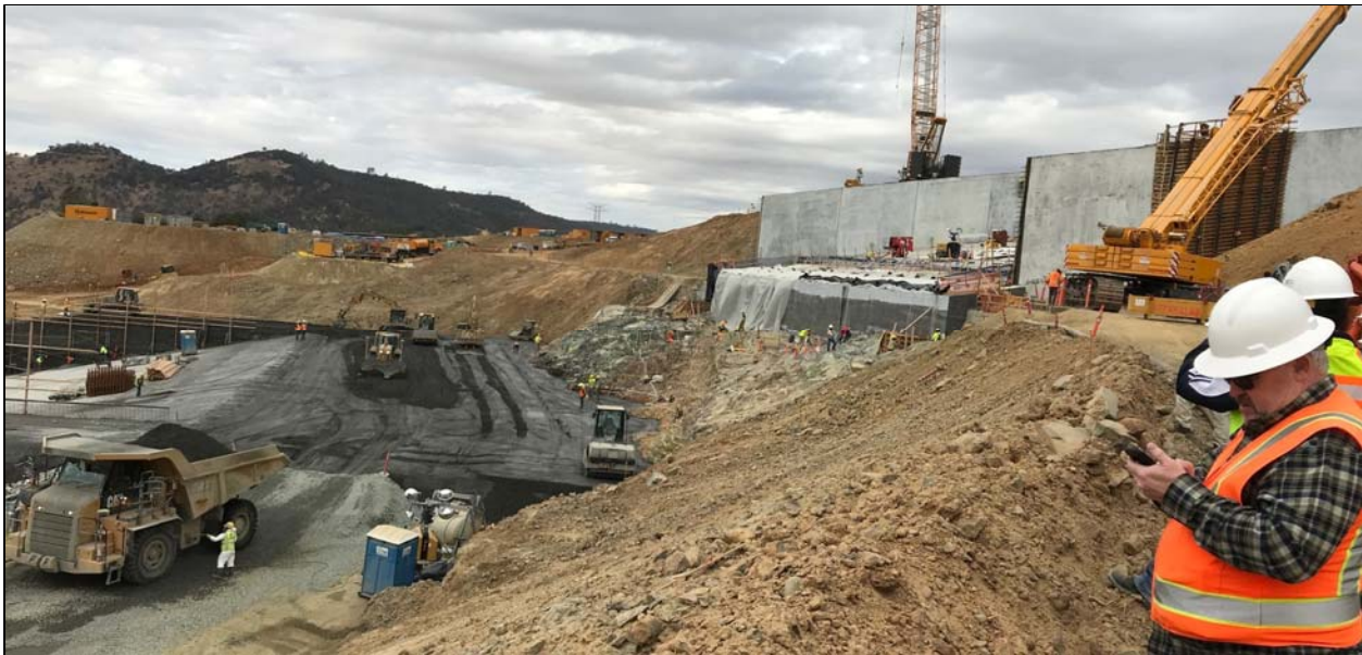
Figure 3. Photograph showing remaining section of the FCO chute to be infilled with RCC (shown at the left) of the main scour hole with the permanent portion of the FCO structural portion shown on the right.
