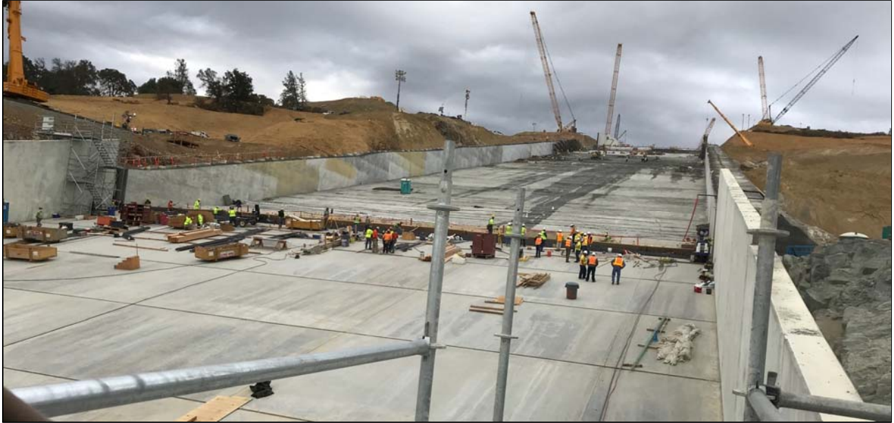
Figure 4. Photograph looking upstream in the FCO Spillway chute at the transition from the permanent structural concrete chute walls and floor slabs (foreground) to the completed RCC sections. The RCC was placed in the areas of the two big scour holes; the RCC filling of the upper scour hole is shown in Figure 3.
