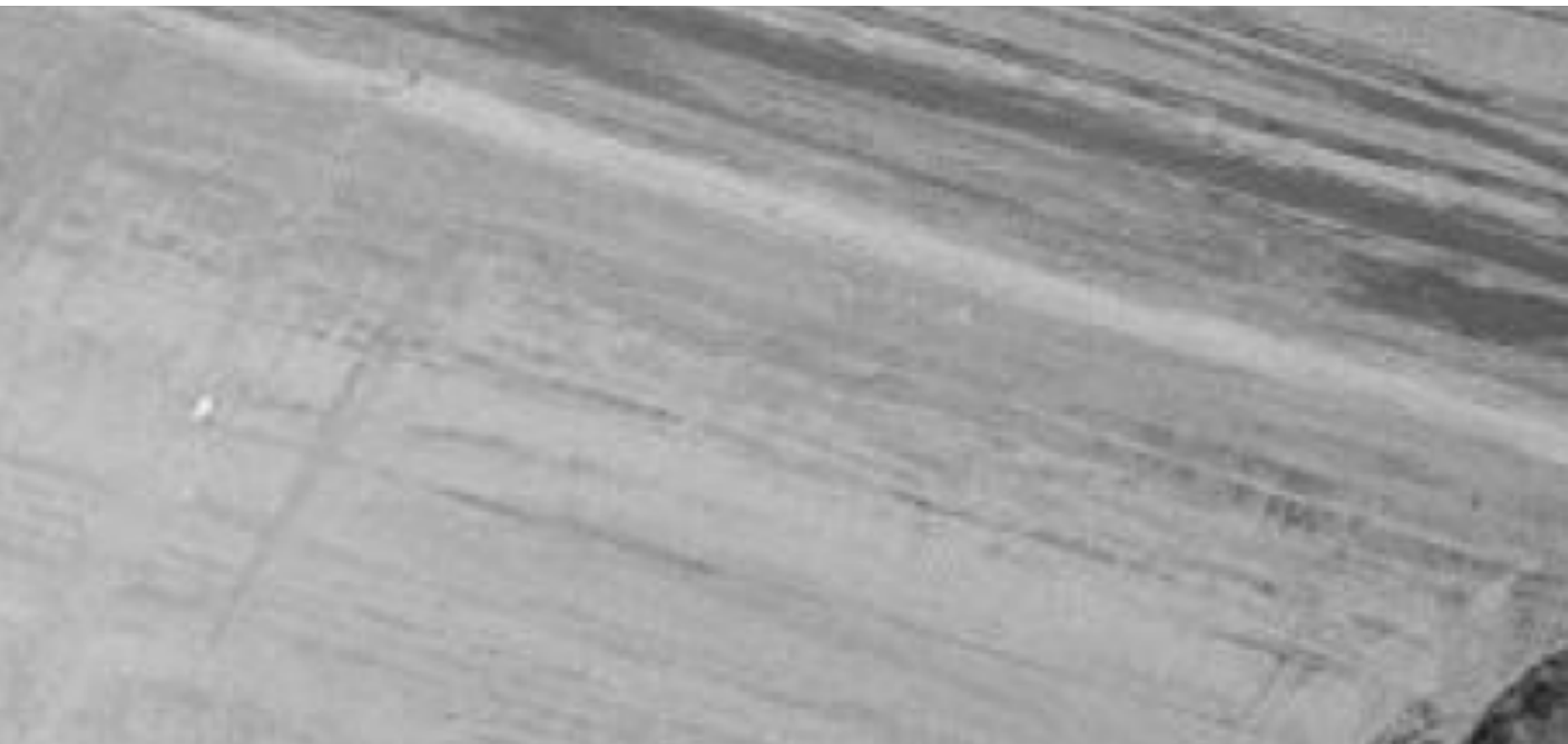
FIGURE 11. Lines of wet areas, ponded water, and erosion rills prior to initial filling of the reservoir in future vegetation area. (Construction photograph taken on November 22, 1966)
