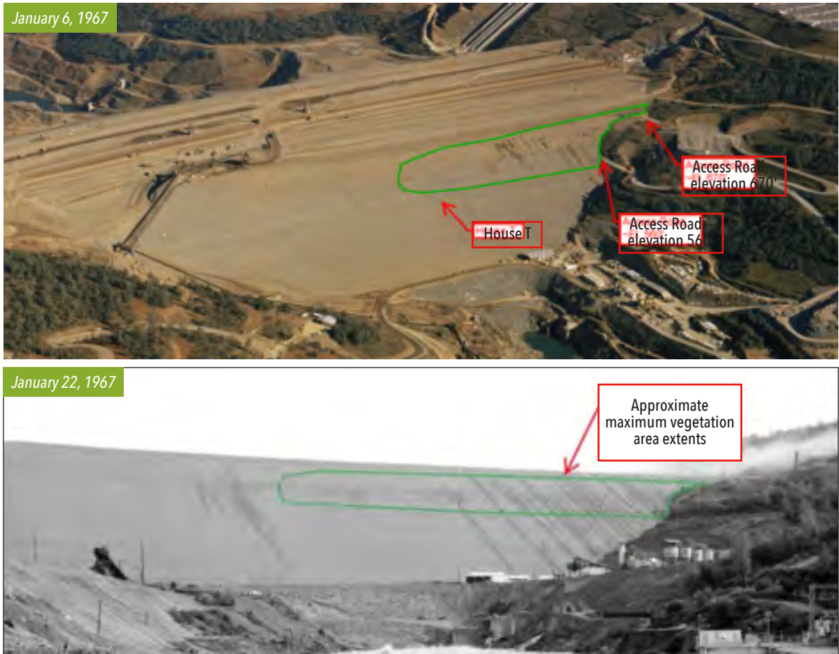
FIGURE 12. Vegetation area showing lines of wet areas and erosion rills prior to initially filling the reservoir. (Construction photographs taken in January 1967)
