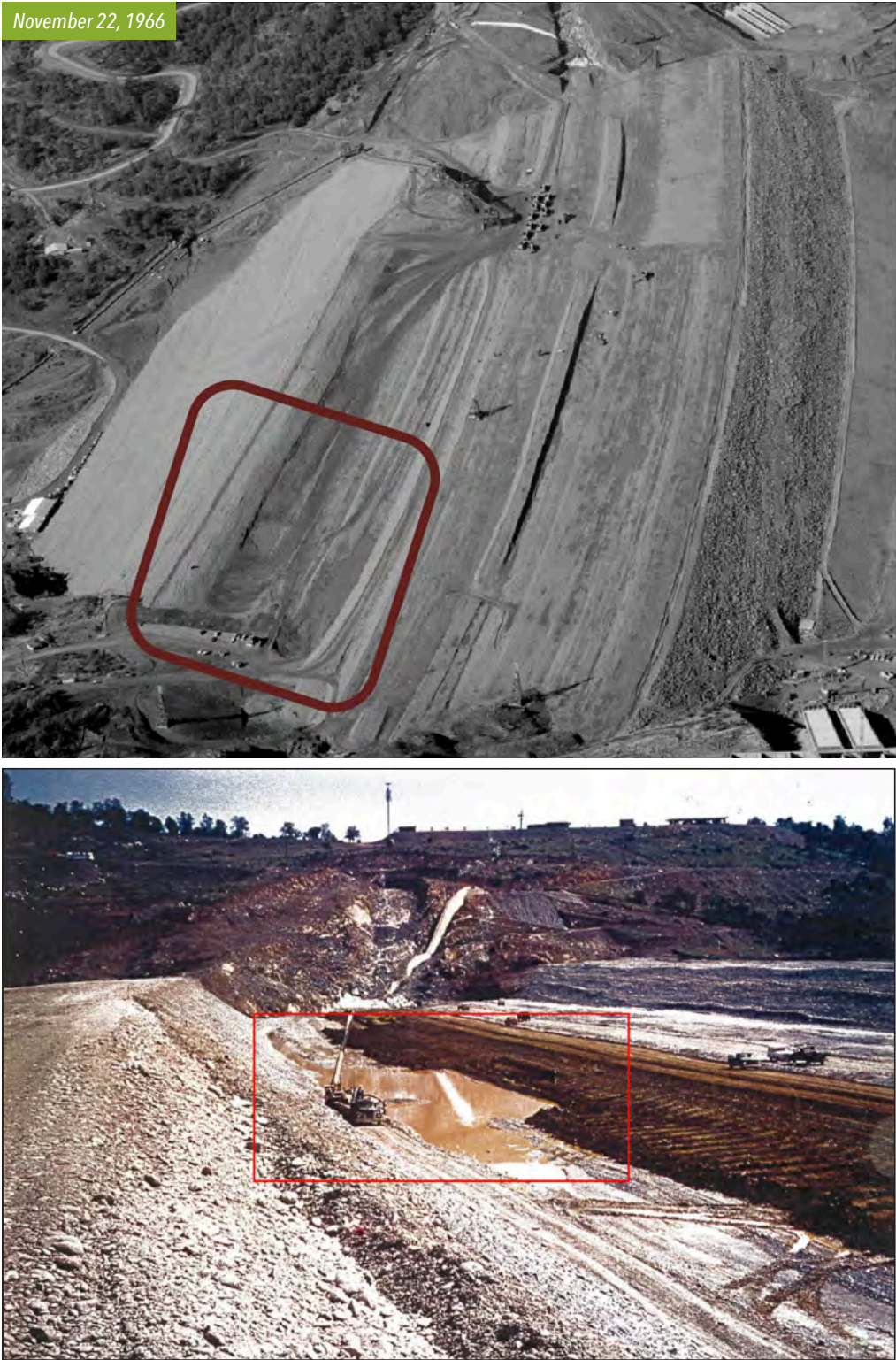
FIGURE 13. Photographs of Ponded Water on the Construction Surface within the Vegetation Area Elevation Range.
