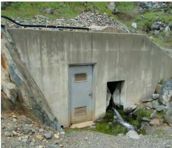
FIGURE 5. View of Seepage Measuring Vault which contains a Measuring Weir, and Interior Low Water Pool Level within Oroville Dam. (Photograph taken on April 22, 2017, when seepage flow was approximately 53 gallons per minute, a relatively low seepage amount.)
