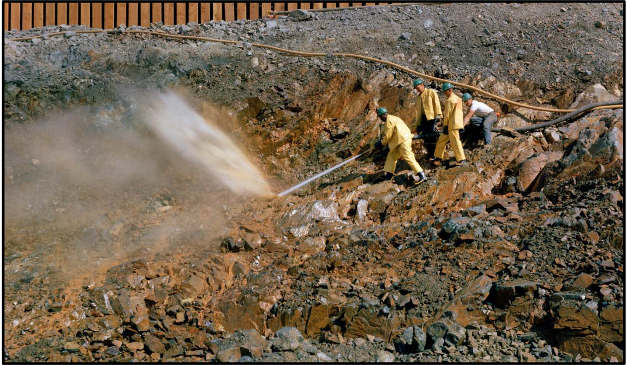
Figure 2: Photograph of Foundation Clean-up Using High Pressure Water Hose in Central Concrete Core Block/Core Area (Photograph taken April 29, 1963, from DWR Photography Files)
