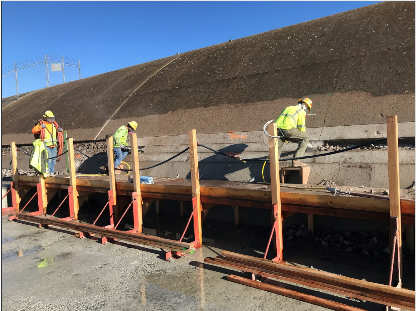
Figure 4. Preparation of the Ogee Emergency Spillway section for placement of Reinforced Concrete Buttress Transition section.
