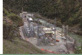
⚡ New Colgate Powerhouse
