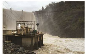
⚡ Narrows II Powerhouse
