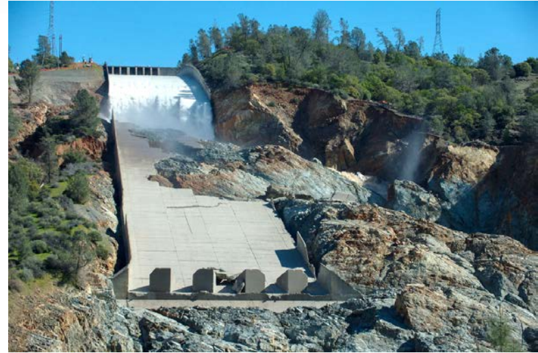
Oroville Spillway damage in 2017. Photo: DWR
